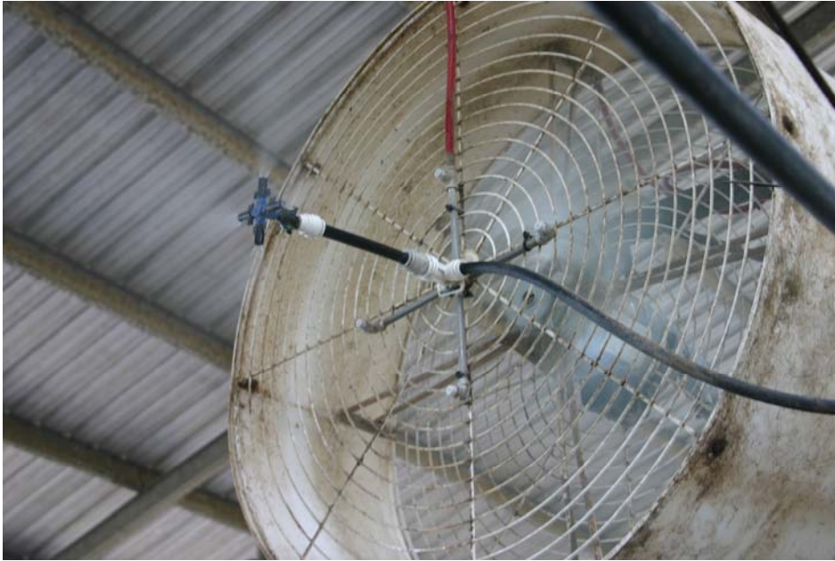
Figure 1. Placement of high pressure and low pressure mister systems on the face of a high-speed, high-volume fan mounted over the feed alley and free stalls.
